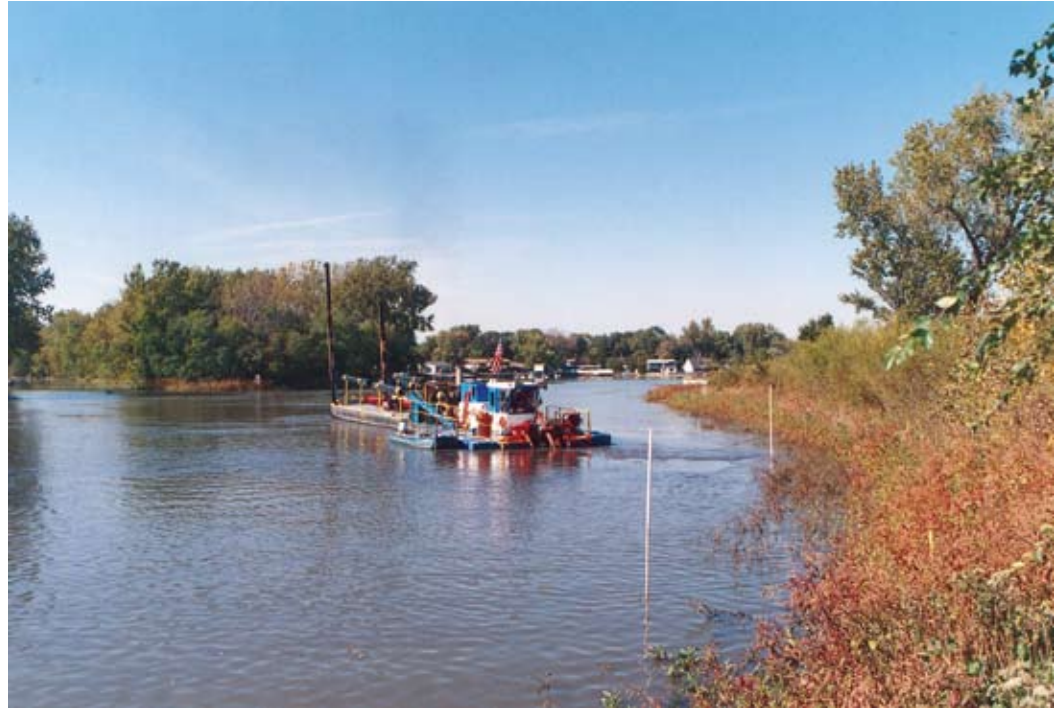
A hydraulic dredge operation in a cove of dense aquatic plants, pumping the dredge slurry to the settling basins.
